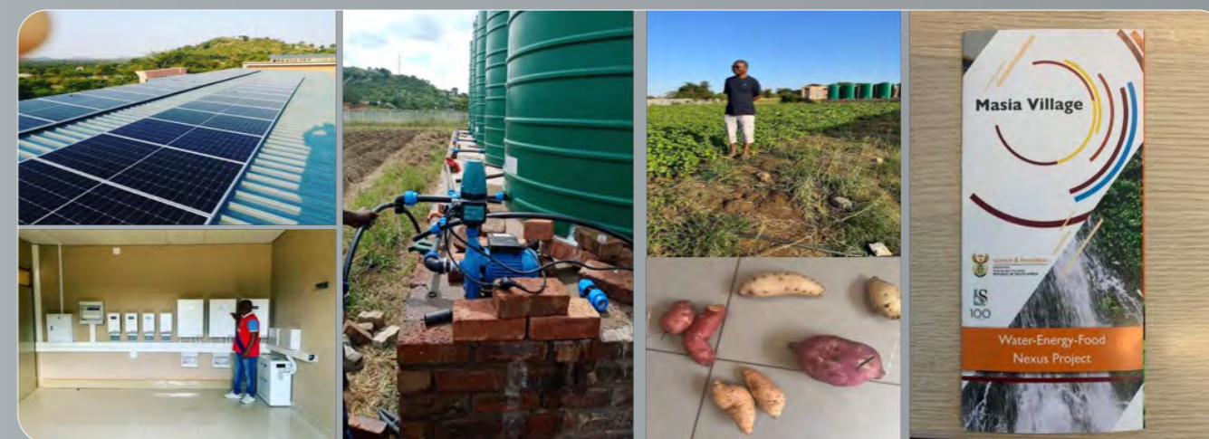
Rooftop Solar PV, battery and inverters. The water storage tanks fitted with water pumping system and the sweet potato field and produce at Masia Village.
